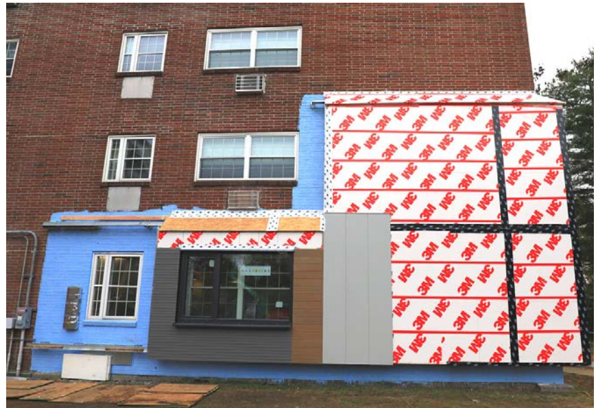
Fairweather Apartments, Salem, during a panel installation demonstration, prior to starting construction.
