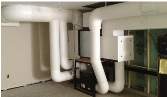
figure 14.16: Photo of completed mechanical system in basement
